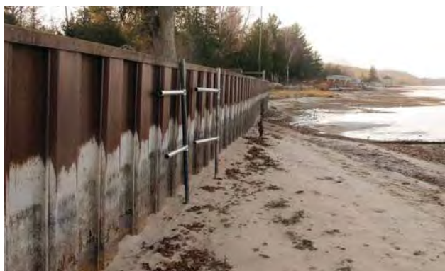
Demonstrating water levels
