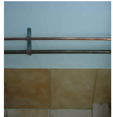
Fixed pipes on brackets
