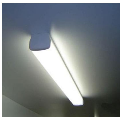
Fluorescent light with shatterproof cover
