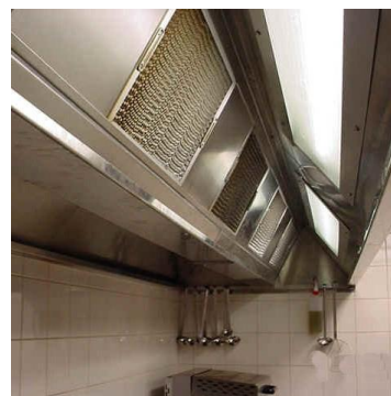
Mechanical exhaust system above cooking appliances
