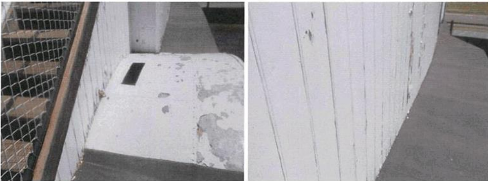
Deterioration visible externally
