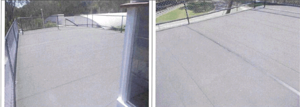
Butynol membrane showing joints, and repairs using 'gaffer' tape where plywood substrate has caused cracking of butynol
