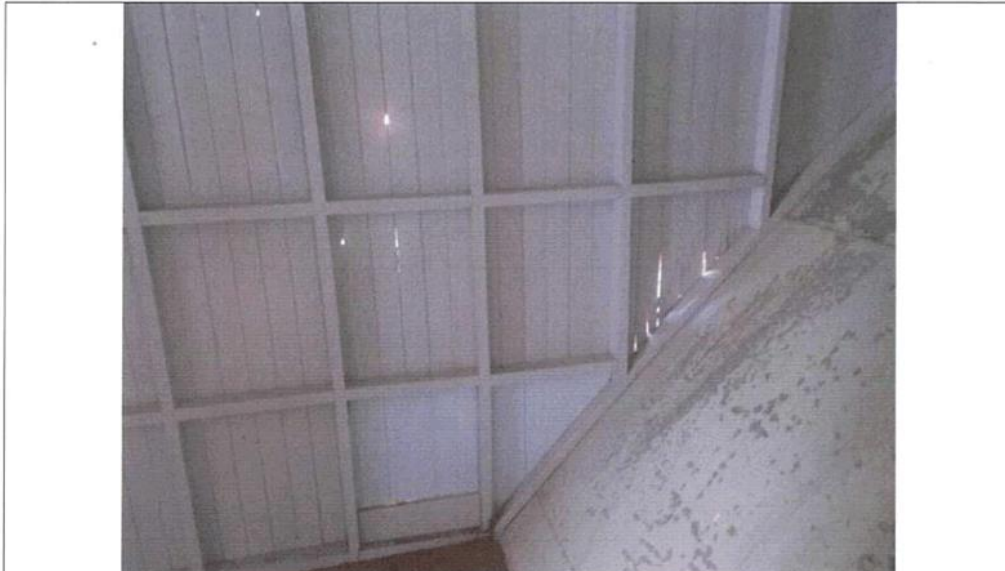
Interior of port side paddle box aft, showing typical damage and running repairs
