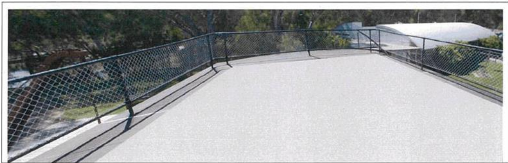
Proposed panel of grey DuroMastic to reduce heat uptake – looking forward from bridge
