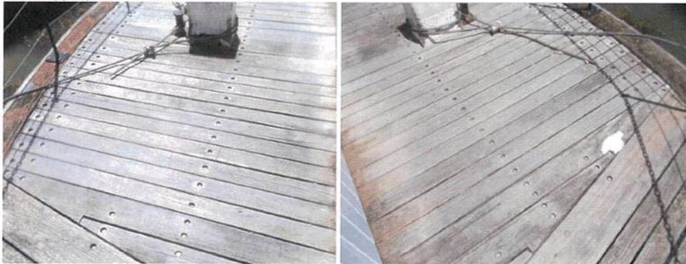
Stern deck showing bolt holes without plugs in central portion
