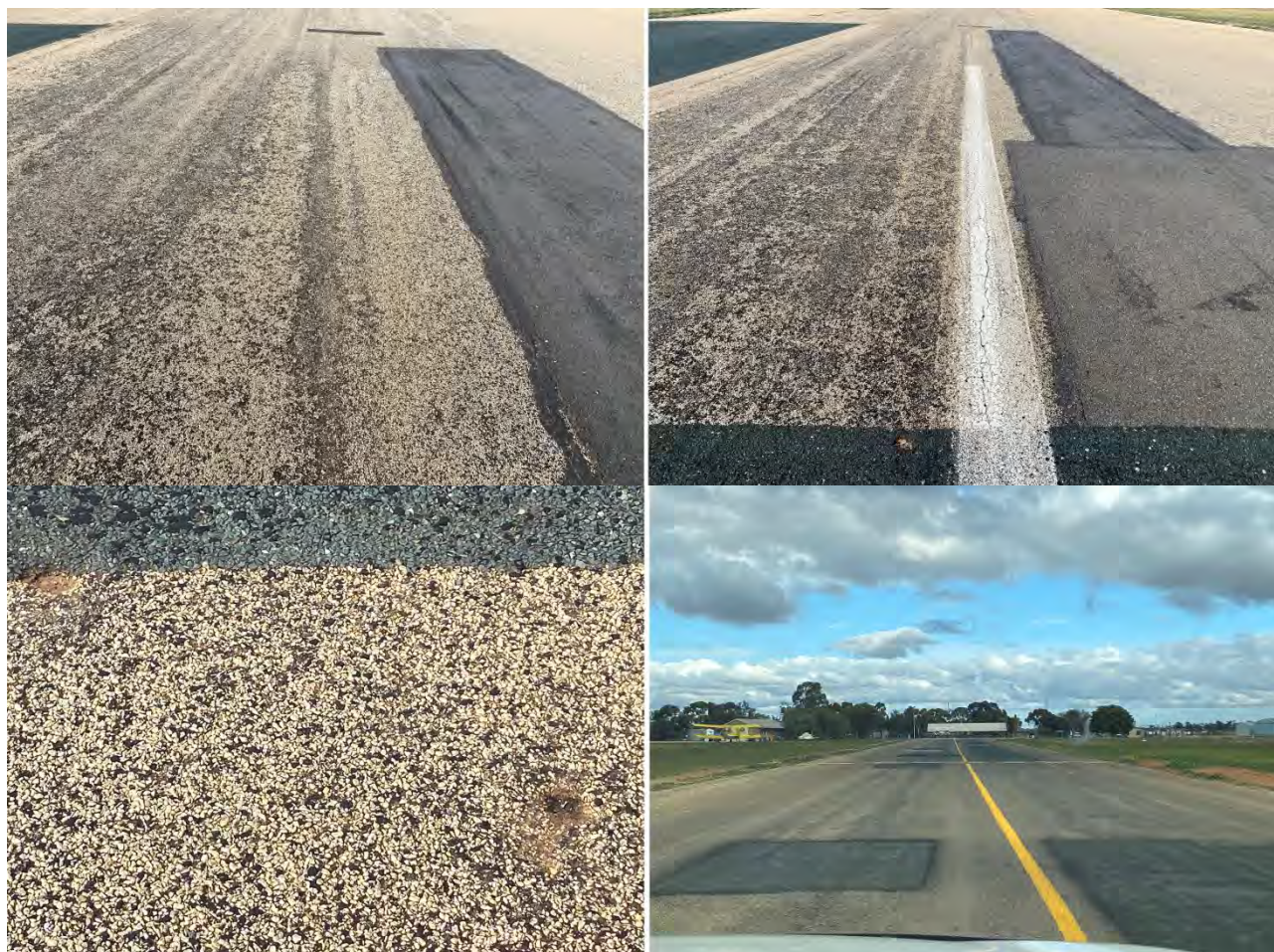
Figure 1 - Cracks on sealed runway & pavement patches.
