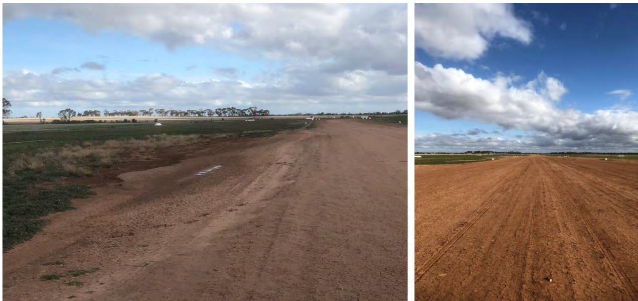
Figure 2 - Natural surface runway / water pooling example.
