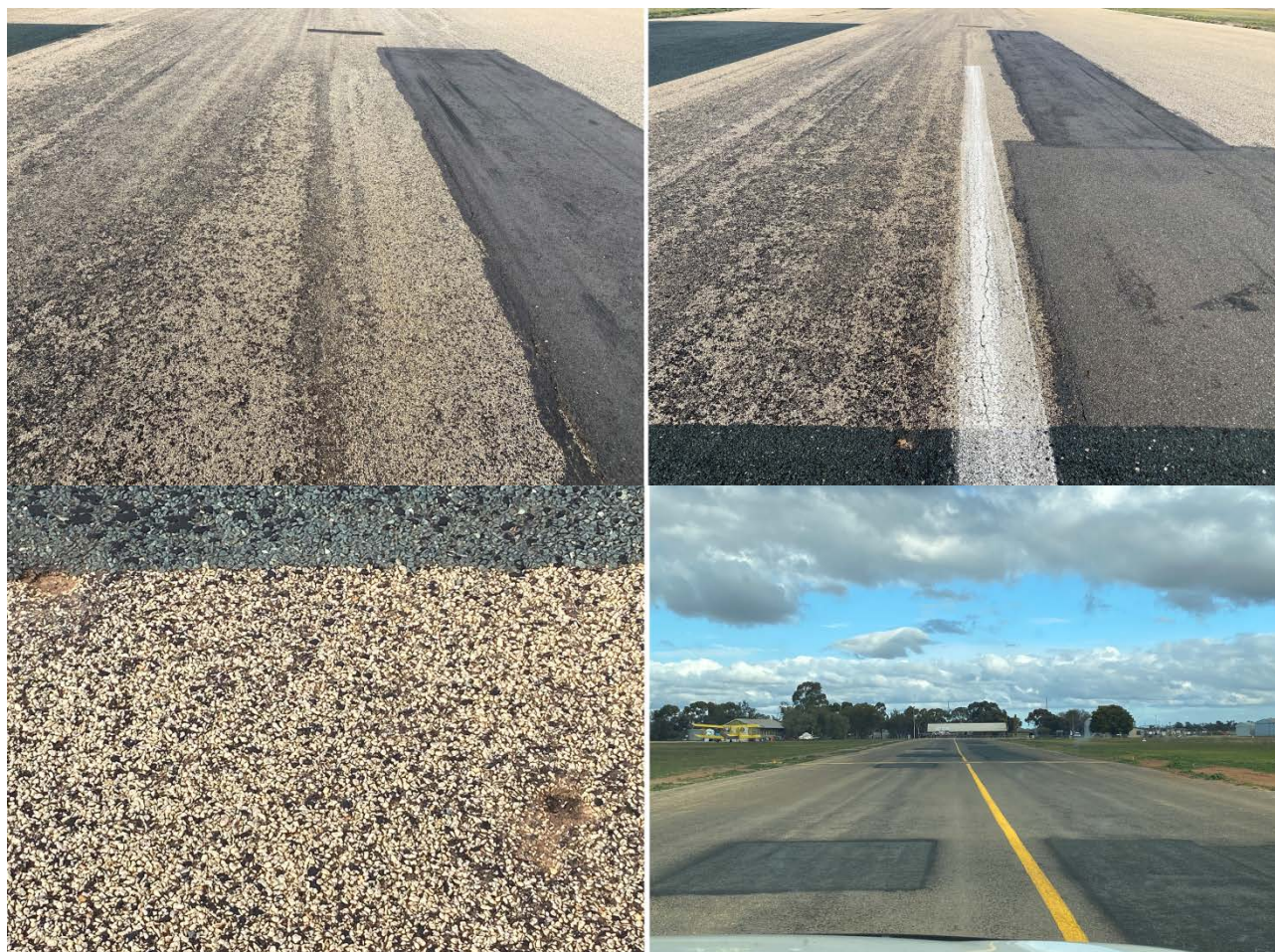
Figure 1 - Cracks on sealed runway & pavement patches.
