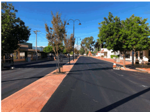
In April 2019, the resurfacing of Perrin Street, Robinvale was completed with asphalt incorporating crumbed rubber, made from recycled tyres. This material comes with a predicted life span of five to 10 extra years, compared with traditional asphalt.
