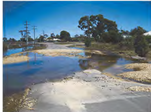
Road damage caused by Tyrrell Creek flooding, Culgoa 2011.
