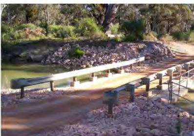
Above: New bridge constructed for access at Mulcra Island. Photo: Mallee CMA.
