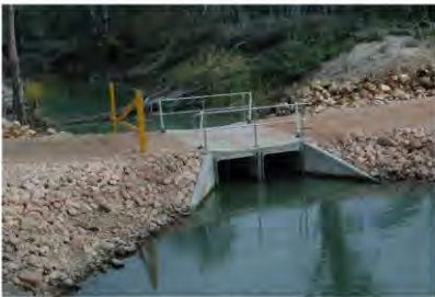
Above: Box Culvert under a bridge at Lindsay Island Photo: Mallee CMA.
